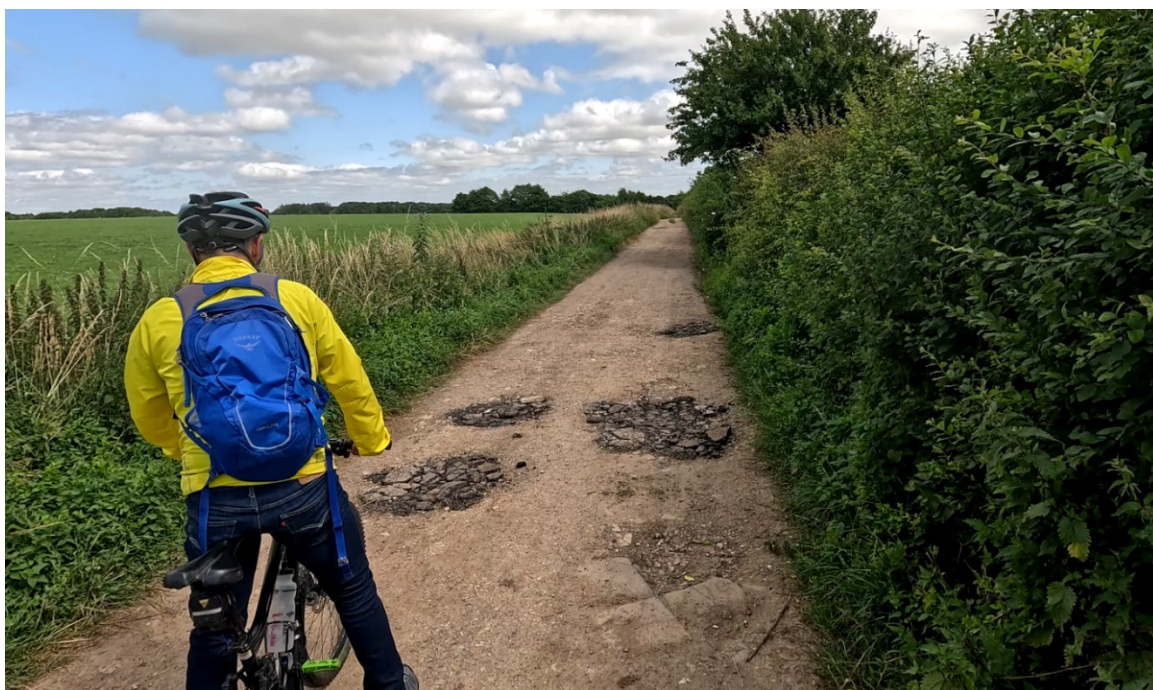
Figure 79 - Poor surfacing on PRow
